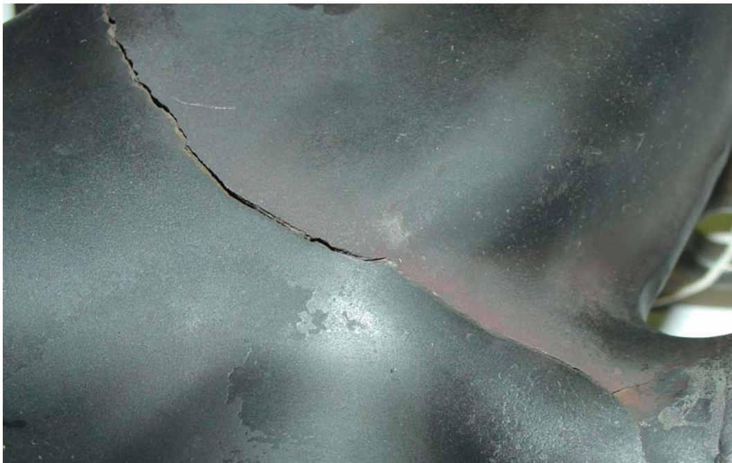
Figure 1 Examples of transition components requiring replacement
